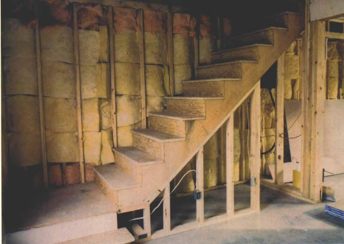
Ready for traffic. With the stair screwed in place and the step to the landing installed, the stair is ready for use by the construction crew. End caps and balusters will be added later during the trim stage. (Note: Insulation scraps made a great sound barrier for the wall behind the stairs.)
